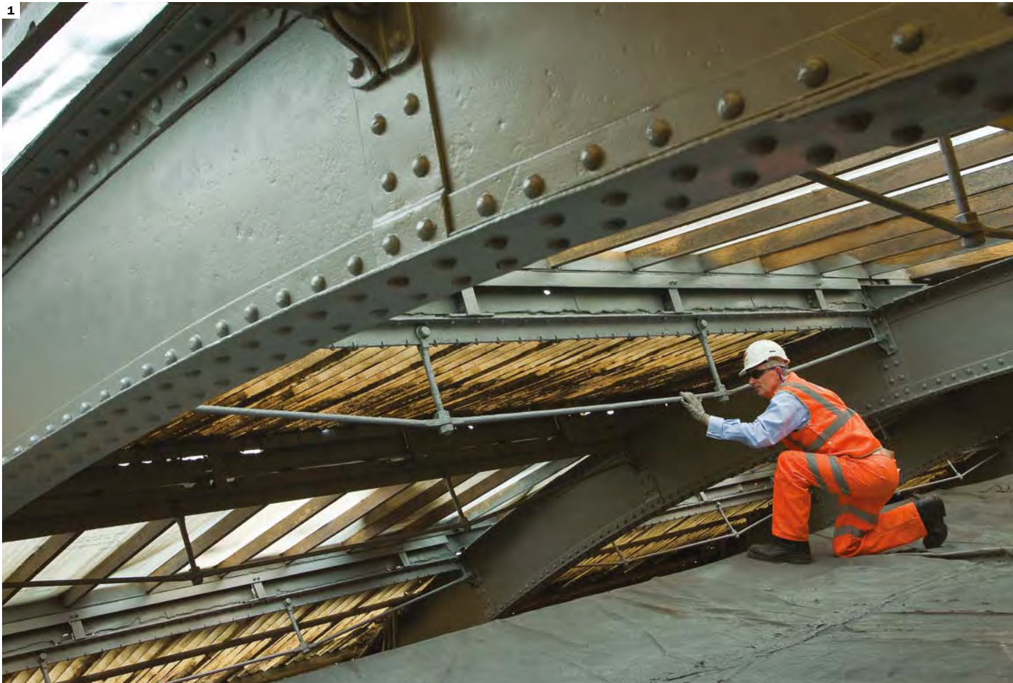
1. King's Cross railway station roof, London, value £27m Kier Construction Construction manager Nick Tindell pictured inspecting the condition of the steel at King's Cross station roof where Kier Construction is erecting a bespoke access deck system for client Network Rail.
