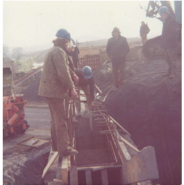
People wearing of Safety Helmets However where's the scaffold?
