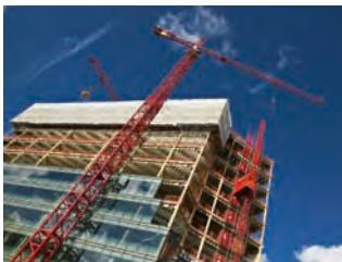
One Reading Central Kier Property Kier Property and Invista Real Estate have created a joint venture to develop this major HQ office campus in the heart of Reading city centre.
