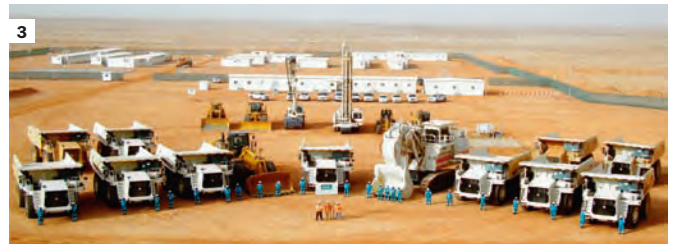
3 Al Jalamid, Saudi Arabia, Kier Construction Plant and equipment ready to commence work on the eight-year contract for Ma'aden of Saudi Arabia to establish and operate an open pit phosphate mine – potentially the world's largest phosphate project. Kier is working in joint venture with its partners, Al-Qahtani (Saudi Arabia) and Comedat (Jordan) on this contract.
