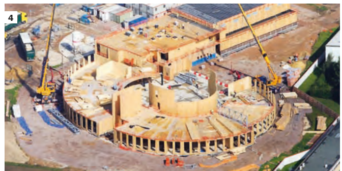
2 Edinburgh Airport, Kier Scotland Kier Airports has completed its first project at Edinburgh Airport as part of the BAA framework. This is a £10m contract to provide a new car hire centre. The Consolidated Car Rental Centre (CCRC), built by Kier Scotland, is one of the first BAA framework projects awarded to Kier since its recognition as a framework partner.
