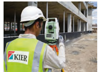
Whitmore High School, Harrow Kier Southern Site engineer Jas Dhaliwal working for Kier Southern on behalf of Kier Harrow Projects which is carrying out a £40m design & build project at Whitmore High School in Harrow. The project is now well under way and completion is due in 2010.
