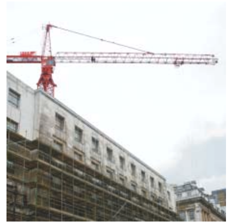
ABOVE A Kier Plant crane working at Whitehall Place for Kier Build.
