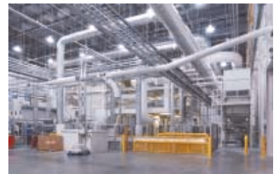
ABOVE New manufacturing facility, Barton on Humber, Lincolnshire for Kimberly-Clark. Kier Northern. 9 10 11
