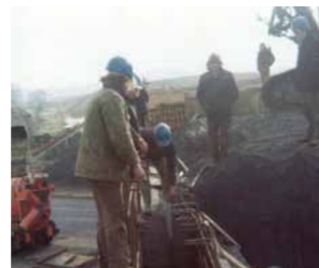
People wearing safety helmets, however where's the scaffold?
