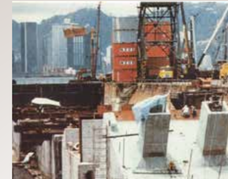
The four precast outfall units being encased in the Hung Hong dry dock
