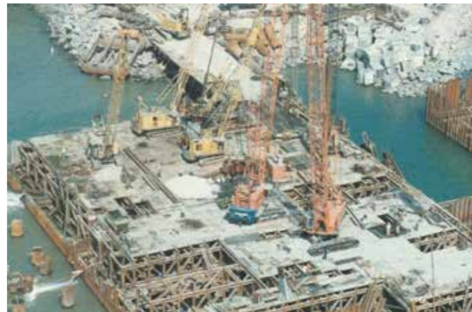
A view of the plant working from the temporary decking. The range of cranes used was from 50-80T capacity and at times there were 5-6 cranes on the deck at one time!
