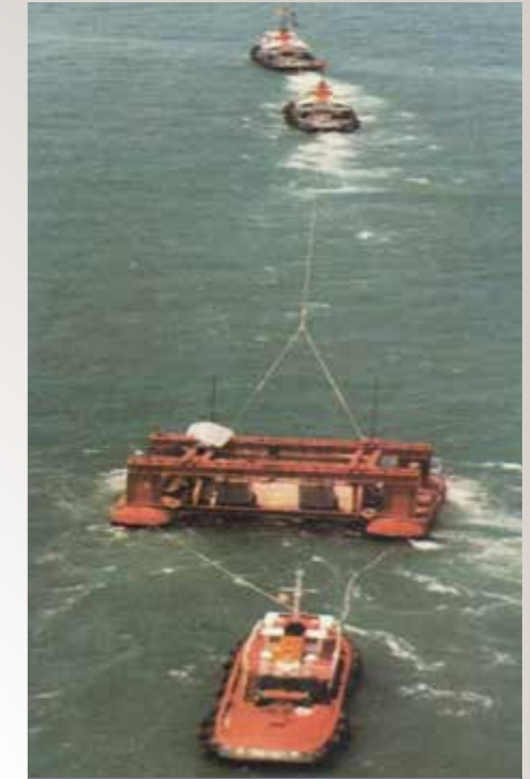
One of the large PC outfall culvert units being towed to site
