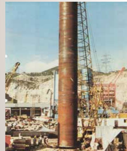
A full length 2.5m diameter permanent pile casing being installed, each 50-60m long (note: the 3.5m diameter temp casing in the ground)
