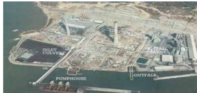
The pumphouse construction: the reclaimed site with the CW project superimposed on it
